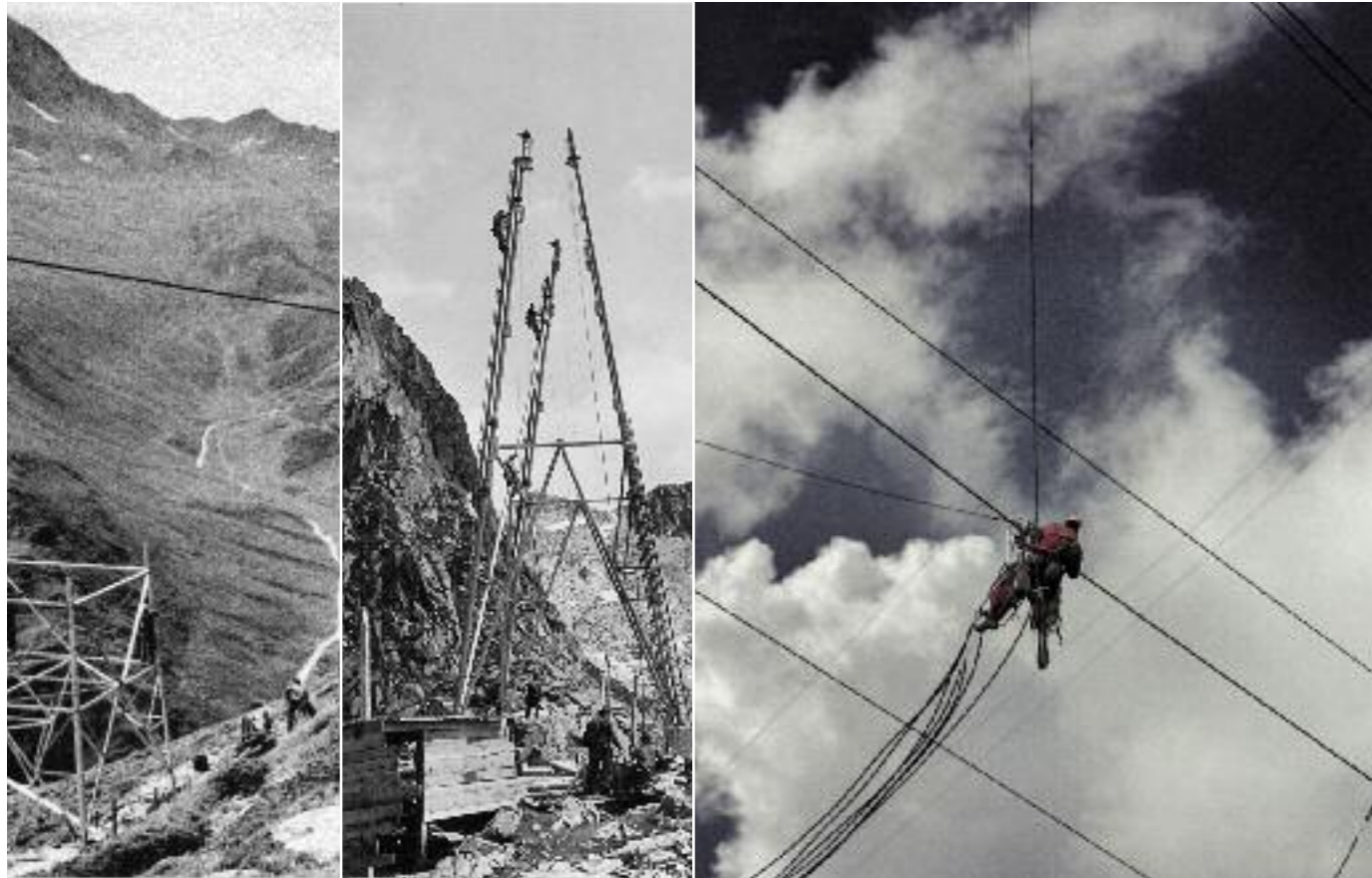
Erection of pylons during the construction of the 220kV Col du Grand St.-Bernard line in 1955
